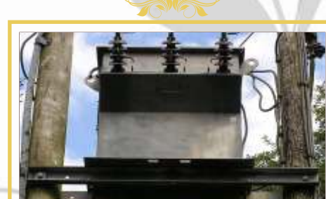
SEPARATE ELECTRIC TRANSFORMER
