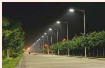
Electric line with Street Light
