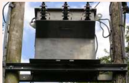
Separate Electric Transformer
